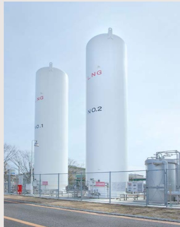
LNG satellite facility and small boiler facility
