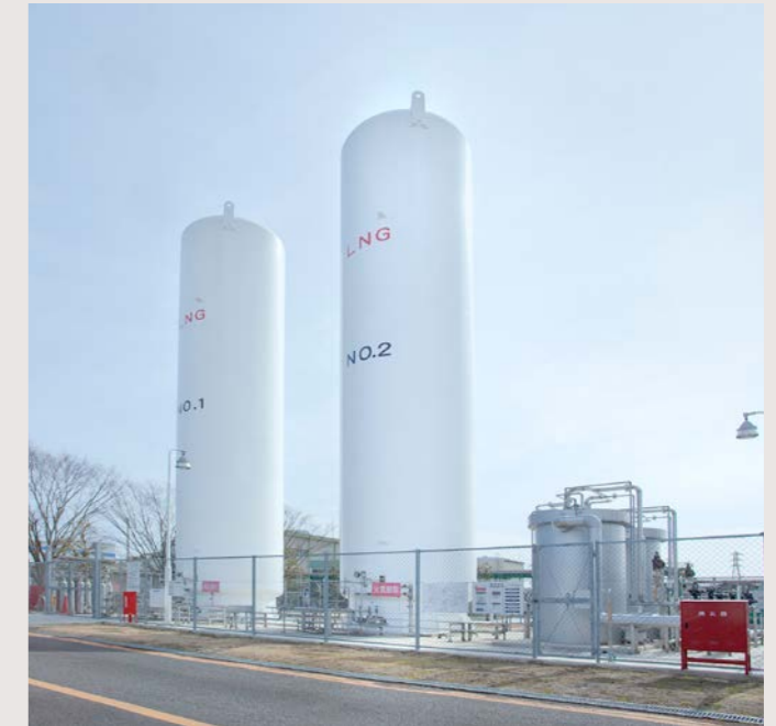
LNG satellite facility and small boiler facility
